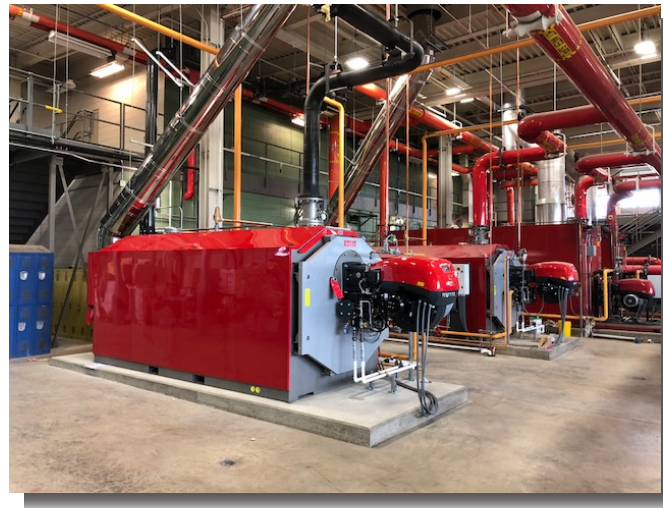
(2) RIELLO RTC 10,000 MBH GAS/#2 OIL CONDENSING WATER BOILERS
