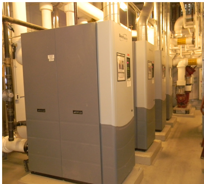
(4) AERCO Benchmark 2.0 Boilers
